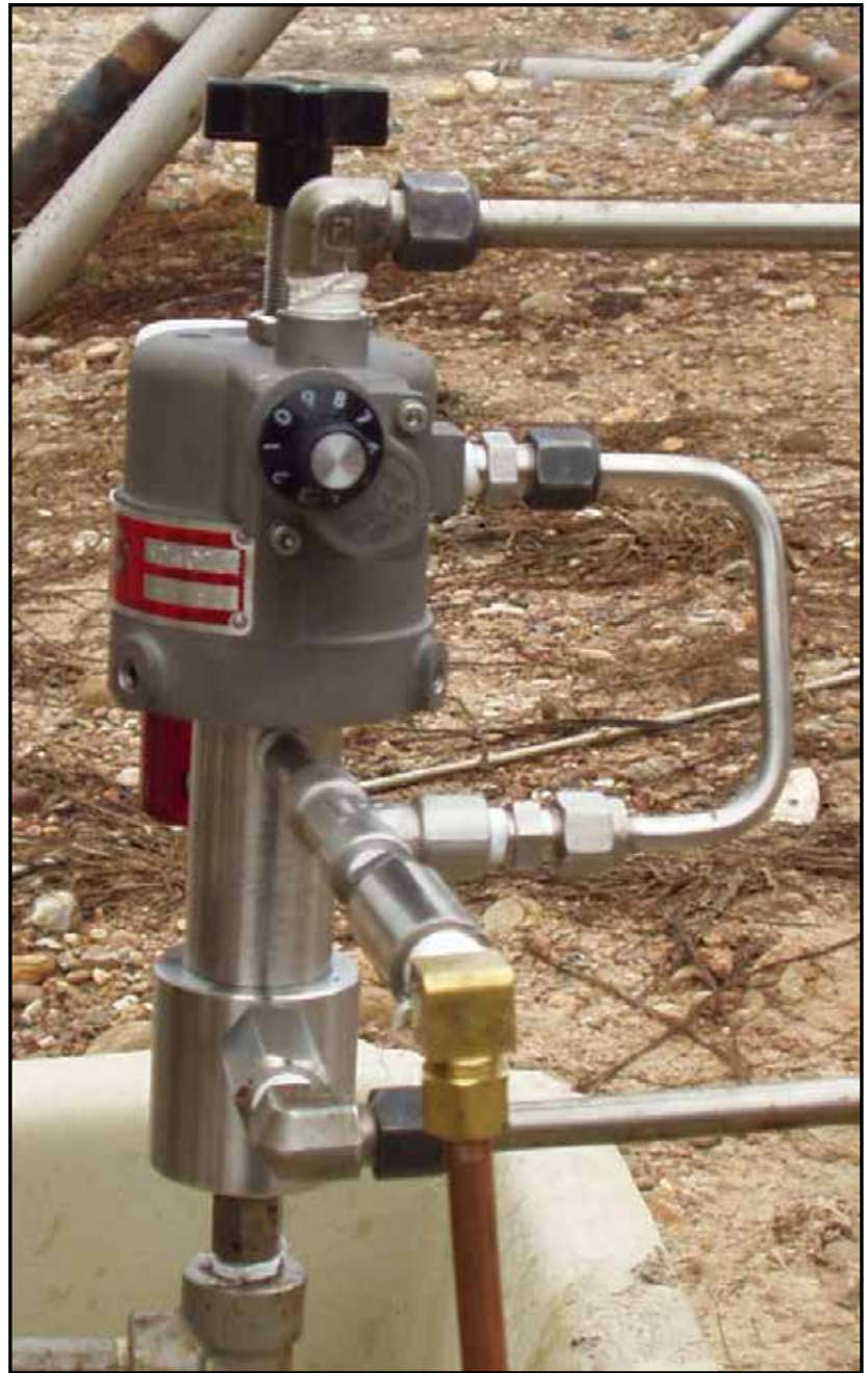
Model 42-402-GS in service Ceramic Plunger with Teflon Graphite Uniseal Pump injecting 10 gallons per day of H 2 S scavenger Exhaust gas recovered to 70 PSI gas line from separator to compressor
